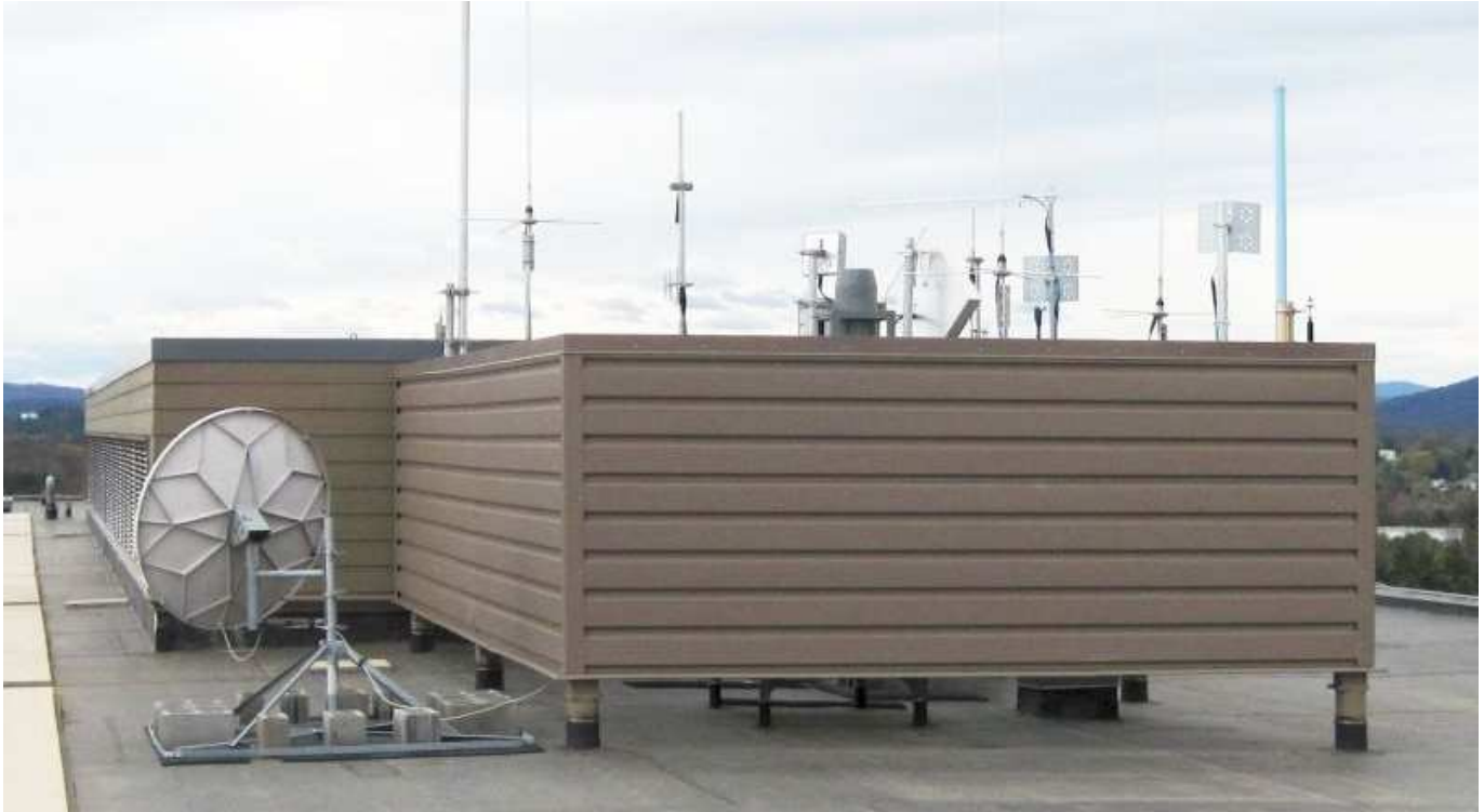
The antenna farm atop the Martha Jefferson Hospital that we have to compete with for space and interference from other services there. (Photo by Ron Richey K4RKA)
